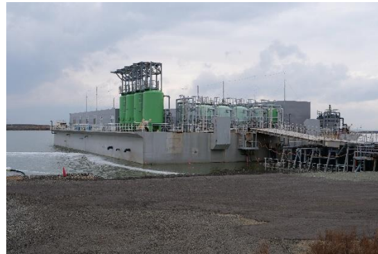
Photo 2-13 Water Treatment Facilities Installed in the Landfill (Reclaimed Land off Osaka Coast)
